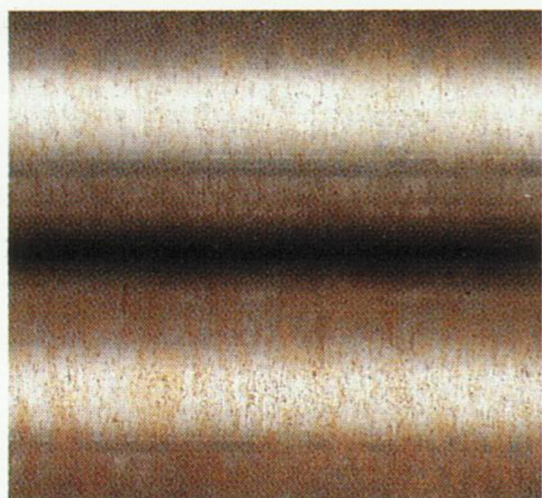
Stainless exposed for 3 weeks to sea spray and groundwater containing sulfides, corrosion so severe that handrails were removed after 3 months.
